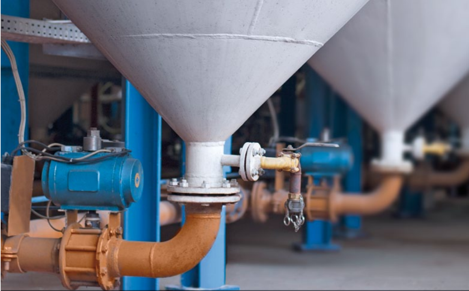
The tank storage area at the Bramsche Industrial Recycling Centre: equipped for the acceptance, sedimentation and fine sedimentation of liquid waste materials
